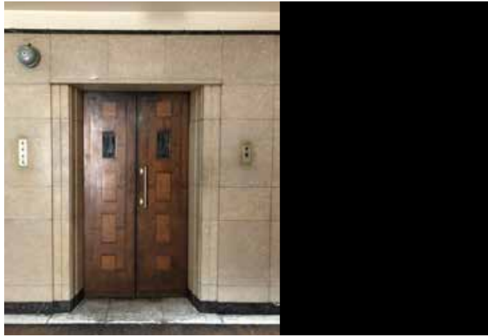
Item description: Lift doors
