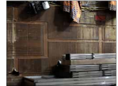
06 Locally replace veneers in sections NTS (cut-out small sections of veneer and reinstate with matching pieces)
