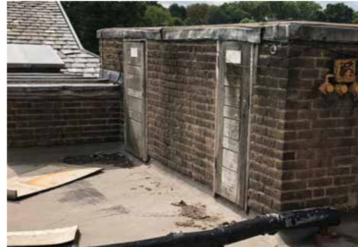
Item description: External timber doors (multiple locations)
