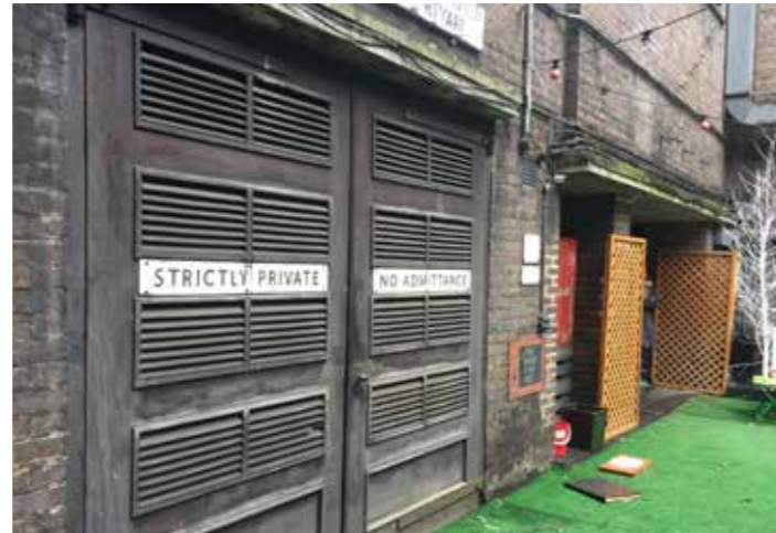
Item description: External louvred plant doors (LG.33/LG.34)
