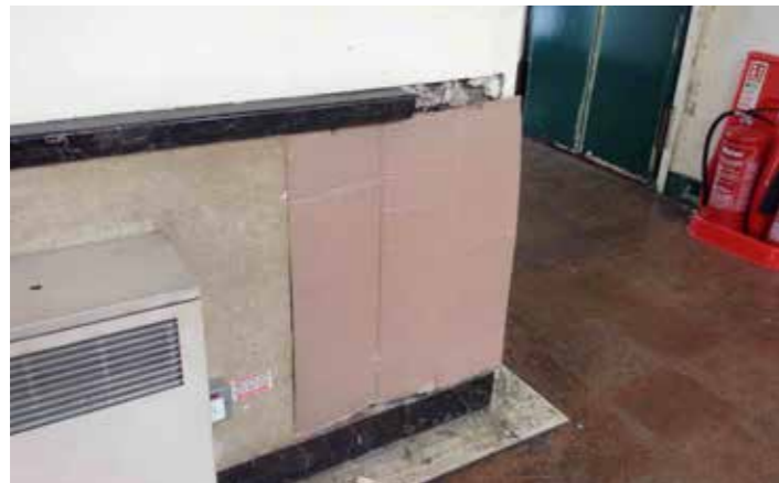
Examples of damage to stone tiling elsewhere in the building.
