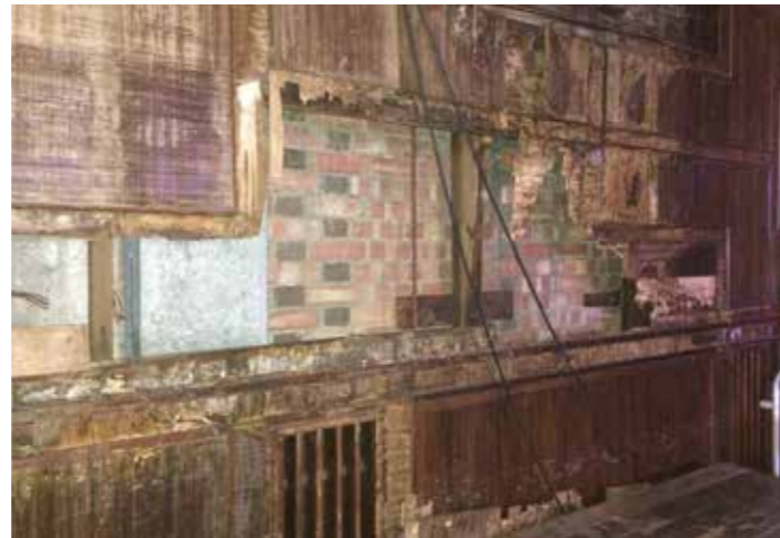
Item description: Timber panelling in the Assembly Hall (Example of panelling beyond repair)
